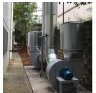
22.5kW and a 15kW Fan
