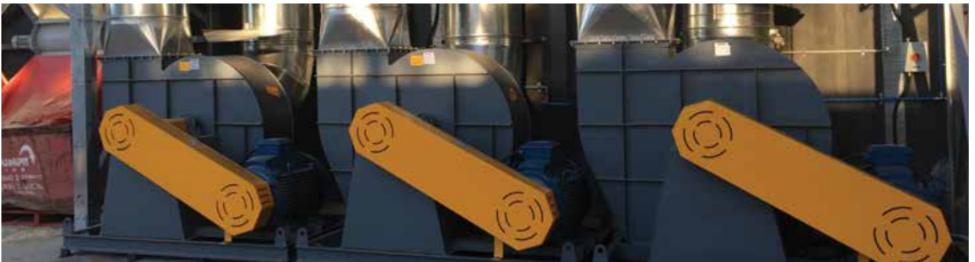
3 x 75kW High Efficiency Centrifugal Fan installed on a large dust collection project in Sydney
