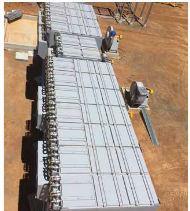
MDC P 130000 (250kW) , MDC PC 72000 (132 kW) and 2 MDC PC 24000 Duct Collectors (45kW) Being installed in an large agricultural application
