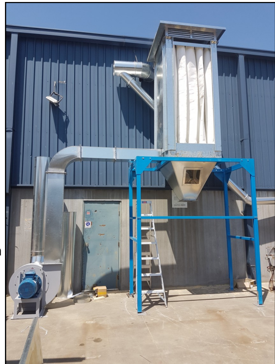
Ezi-Duct eCono 8000 HRVS Installed in a Melbourne Truss Manufacture . The customer is very happy with the units performance and simplicity of emptying the waste bin
