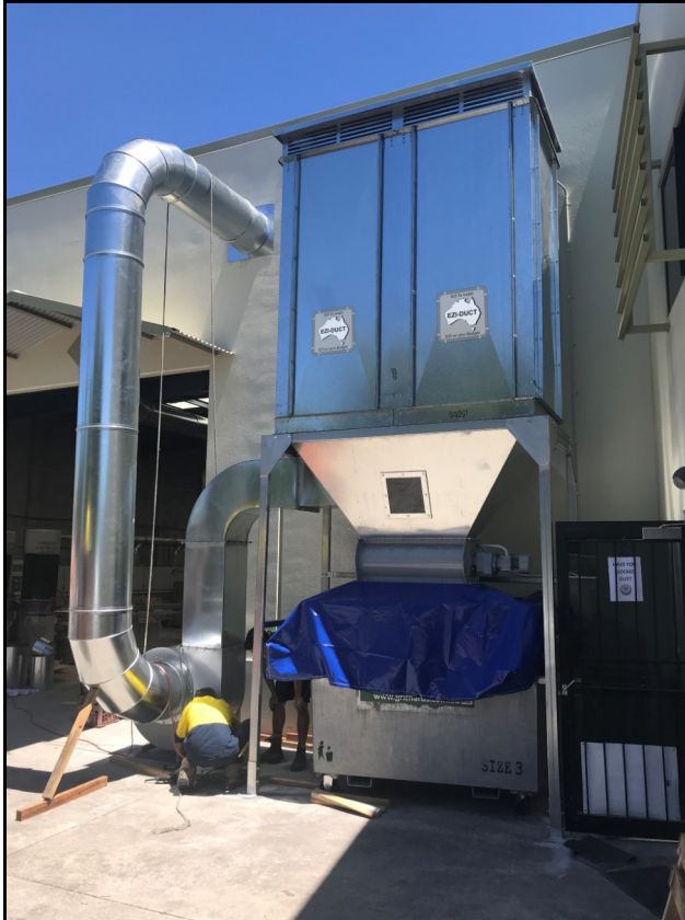
Ezi-Duct eCono 15000 HRVS Installed in a Queensland Kitchen Manufacturer. The customer is very happy with the units performance and simplicity of emptying the waste bin
